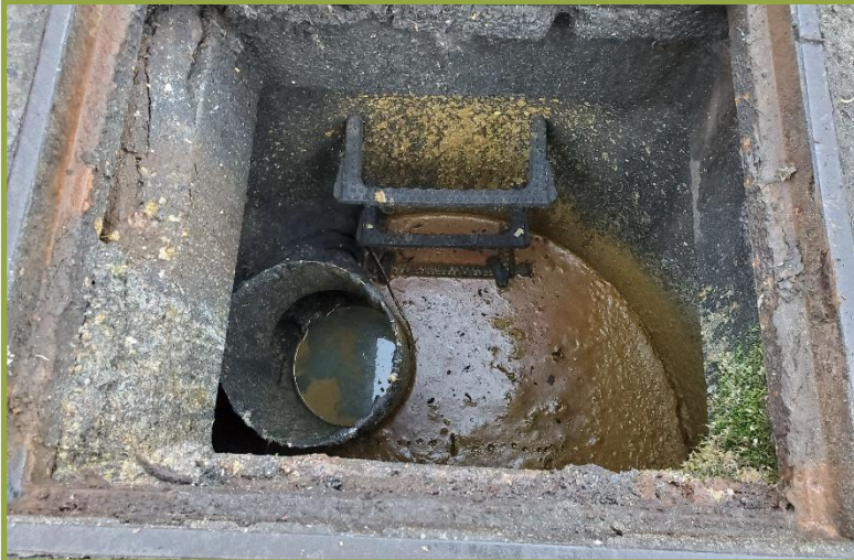
Detected illicit discharge of food waste
