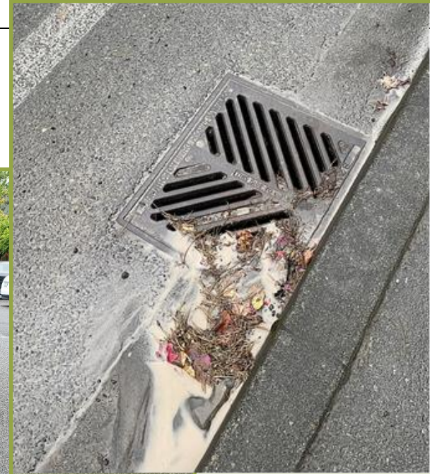
Detected illicit discharge of sediment debris
