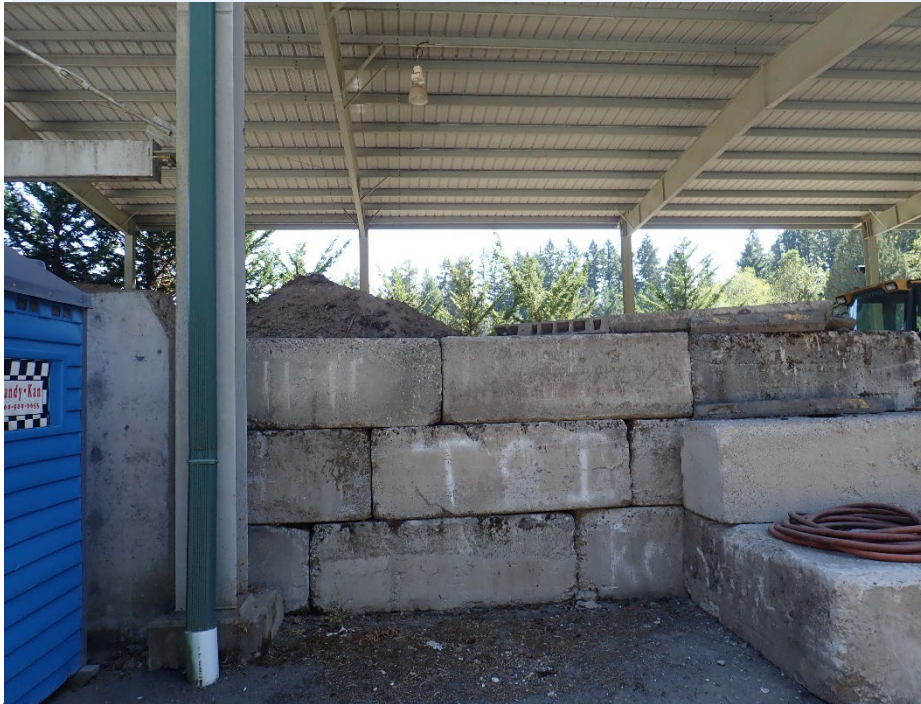
Photo [7] Description: Soil stockpiled above six-foot cement stem wall containment.
