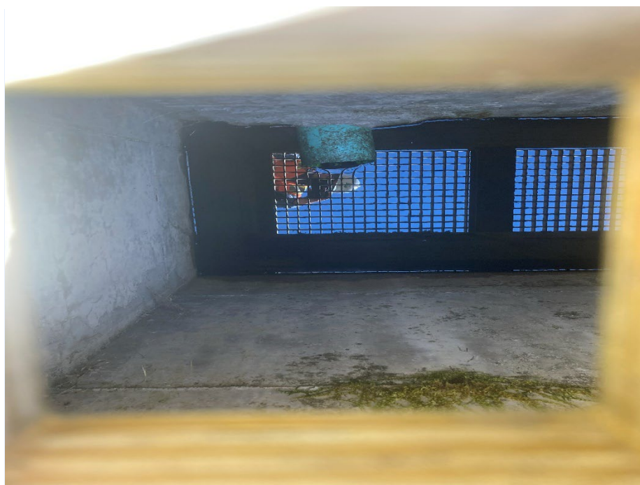
Photo [22] Description: Sand filter inundated with water.
