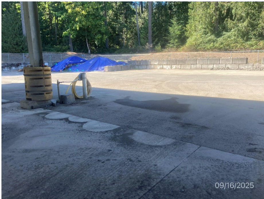
Photo [8] Description: Evidence of track out leaving the decant facility to rest of yard. Moisture on ground was due to street sweeper filling up water tank
