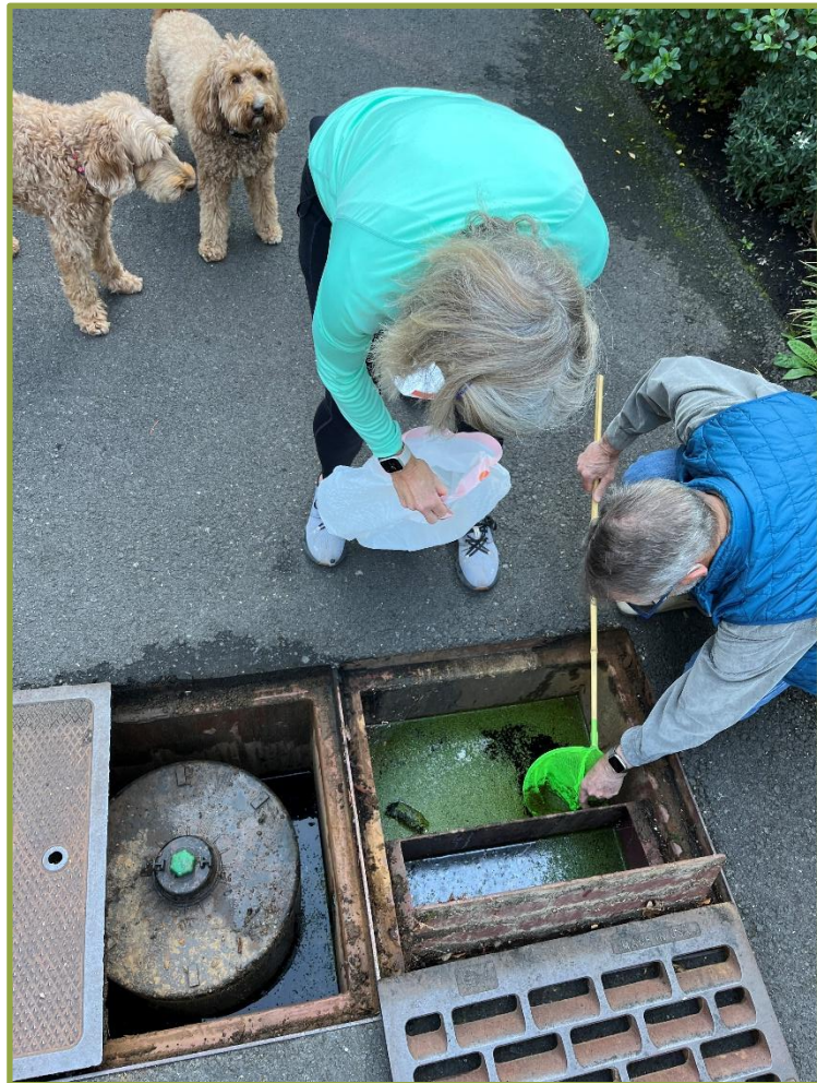
Inspection and maintenance activities conducted by the owners/operators of a City regulated stormwater treatment system
